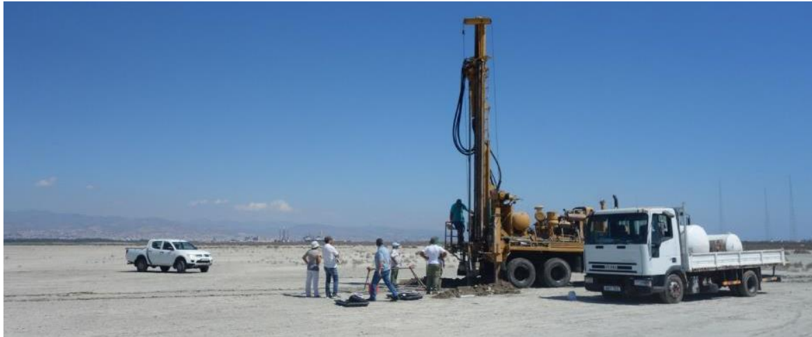
Figure 2 – Mechanical corer (Schramm Rotadrill) from the Company GeolInvest (Cyprus) under the supervision of Andreas Shiathas (Eng. Geologist – Manager Director)
