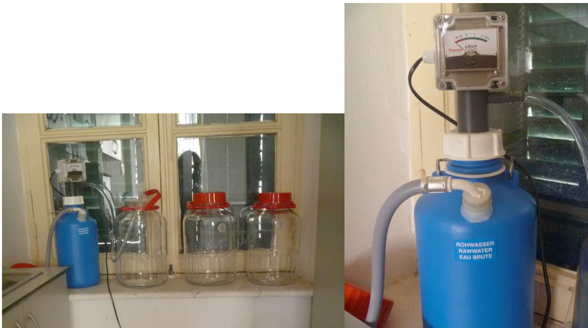
Figs. 7-8: Photographs of the “DI 750” water deionizer unit installed in the Conservation Laboratory in Nicosia. Photographs courtesy of Cassy Cutulle, 2016.
