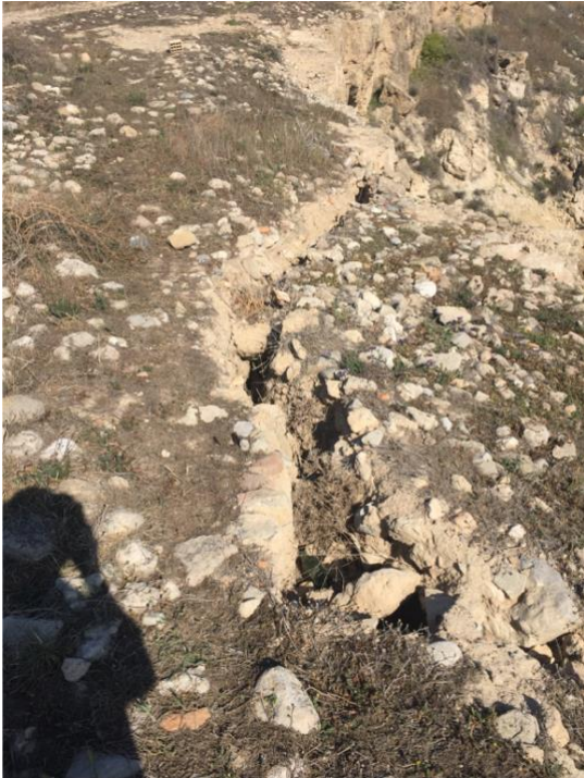
Fig. 10. Erosion from the shore line of Akanthou (Photo taken by Mehmetcan Soyluoğlu)
